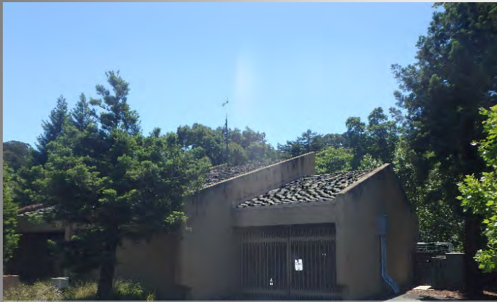
SOQUEL PUMP STATION (At Nob Hill)
