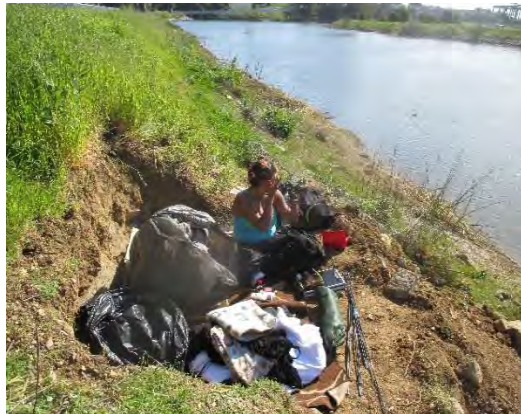
Levee damage caused by illegal camping
